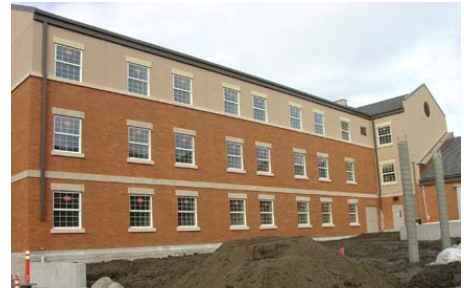
The first of a number of barracks construction projects to incorporate sustainable design
